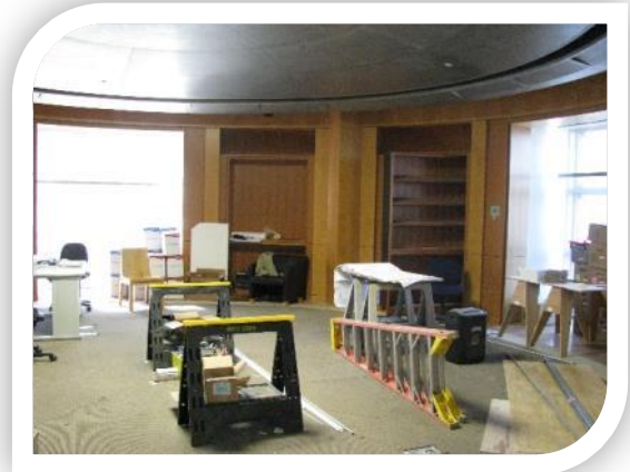
Bridge at The Main Literacy Centre San Francisco Public Library - under construction
